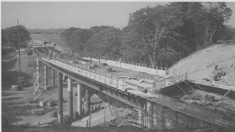
Work on the £8.5m Prudhoe by-pass is ahead of schedule and should be completed by the end of December. This picture shows progress on the bridge which will take traffic over the wooded valley of the Stanley Burn, near Bradley Hall Farm.
