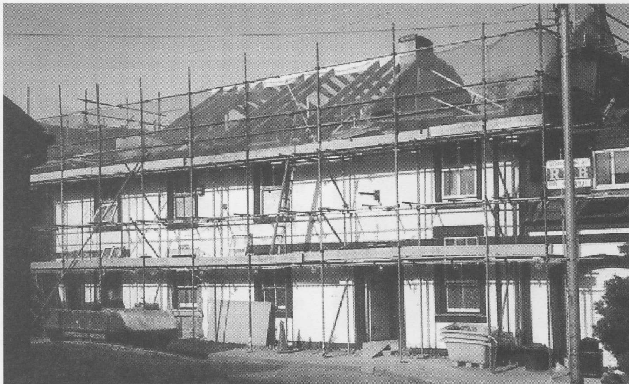
Compare this picture taken several months ago while work was in progress on modernising the Black Bull Inn, with the impressive completed premises which you can now see - and enjoy using - on the Main Street.
